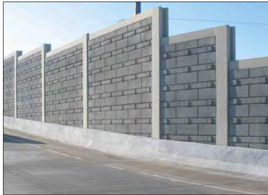
Local Example of a Noise Barrier Wall 1-40 North Little Rock View from the Highway Side
