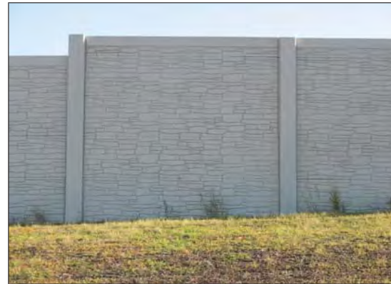
Local Example of a Noise Barrier Wall 1-40 North Little Rock View from the Community Side
