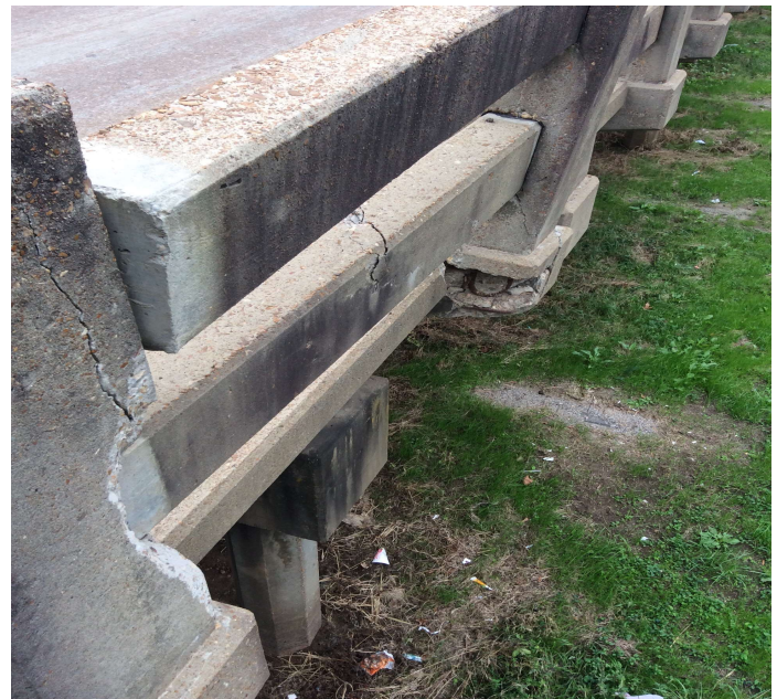
PHOTO 2 Description 1st and 2nd concrete post of left at Span 4 is broken & lower concrete rail is cracked, top rail is off post on one end.
