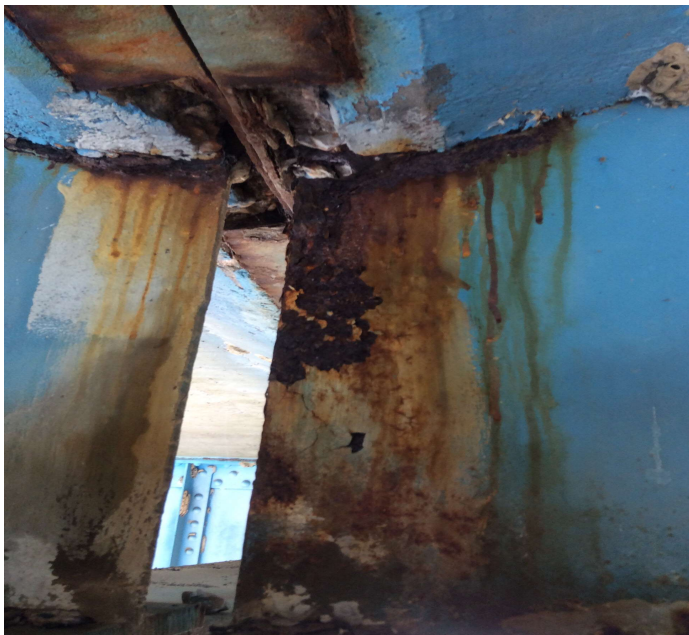
PHOTO 1 Description Rust with section loss and holes in web of stringer #1 at Spans #1 and #3.
