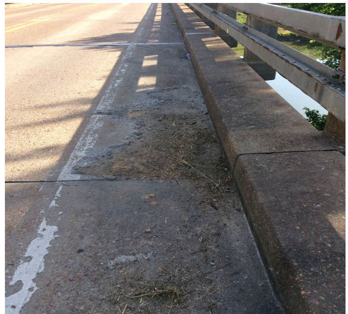
PHOTO 2 Description Spalls to Deck at most spans.
