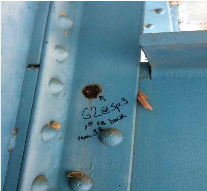
PHOTO 1 Description Sheared rivet at Floor beam connection at Girder #2 at Span #3. 1st floor beam back from 3B
