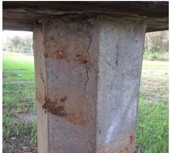
PHOTO 2 Description Vertical cracks with delaminated area to top of Pile 1 at Bent 6.
