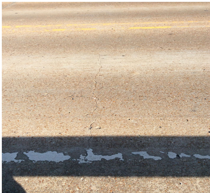
PHOTO 1 Description Unsealed cracks to Deck at all spans.
