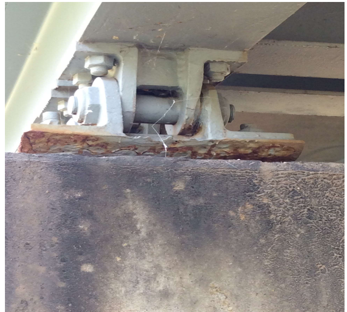
PHOTO 2 Description Heavy section loss to all moveable bearings. (EOS 7)
