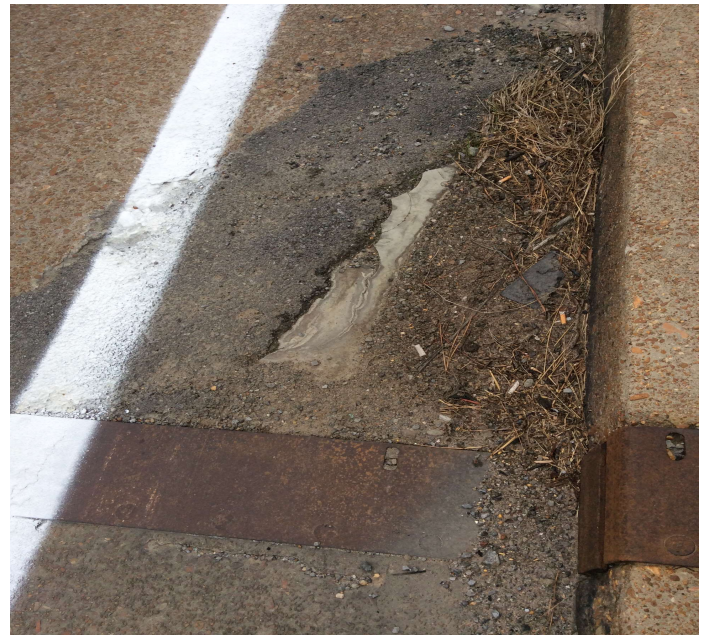
PHOTO 2 Description Spalling & epoxy patch failures in right gutter line Spans 2, 5, 7, & 10.
