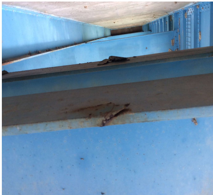
PHOTO 1 Description Floor beam 1 has a crack in top Flange at Span 5.
