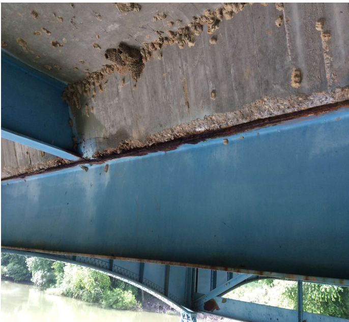
PHOTO 1 Description Rust with section loss to top flange of Floor beams.
