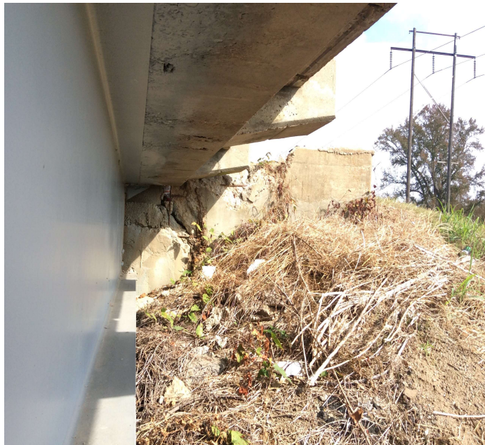
PHOTO 1 Description Typical of Right & Left Wings at Abutment 2 cracked and spalled. (Right at Abt. 2)
