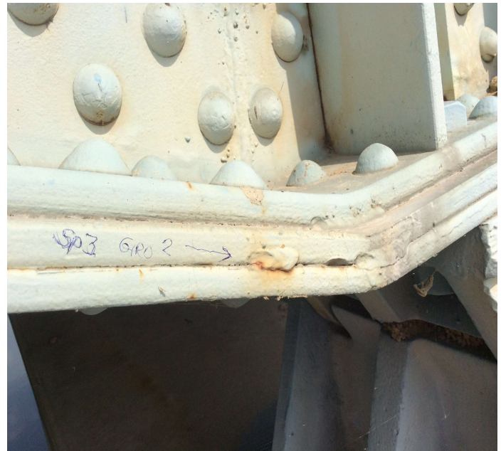
PHOTO 2 Description Cracked tack weld on outside of Girder 2 between bottom flange & cover plate @ end of Span 3.
