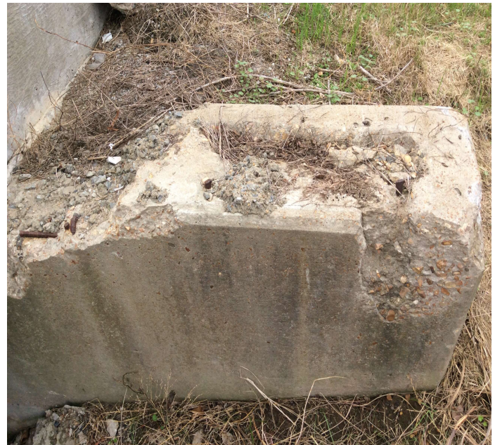
PHOTO 2 Description Typical of heavy spalling to Left & Right wings at Abutments 1 & 2. (Left Wing at Abt. 1.)
