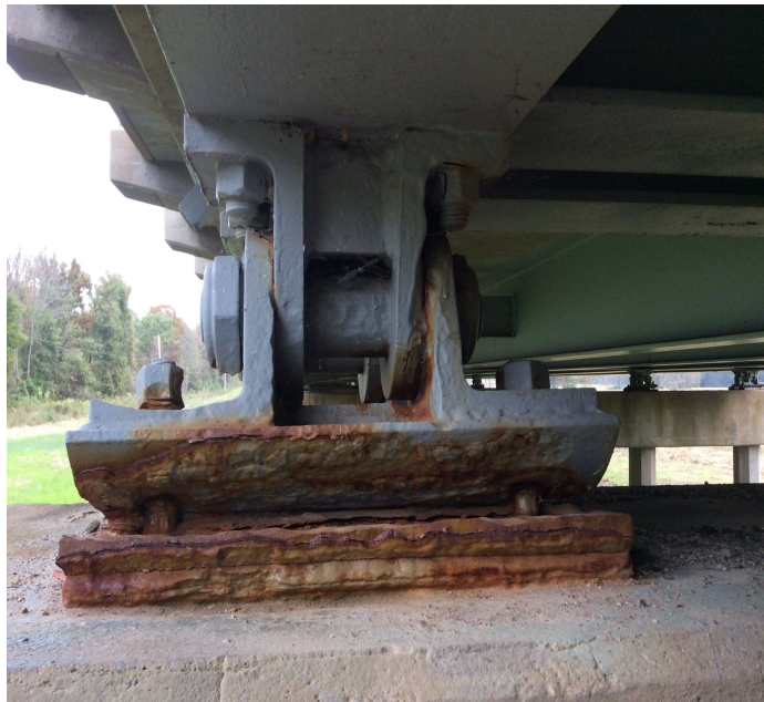
PHOTO 1 Description Heavy section loss to all moveable bearings Section loss to several anchor bolts and nuts with some bent or missing.
