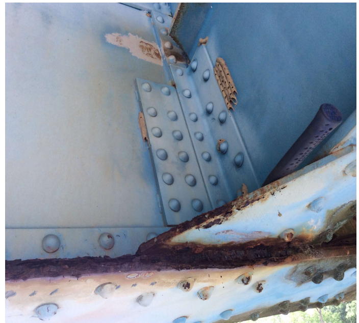
PHOTO 2 Description Heavy rust with section loss to bottom Flange of Girder 1 at Pin & Hanger 3B.
