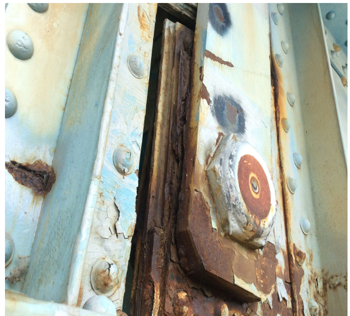
PHOTO 2 Description Girder 2 Pin & Hanger assembly 5A. Pack Rust
