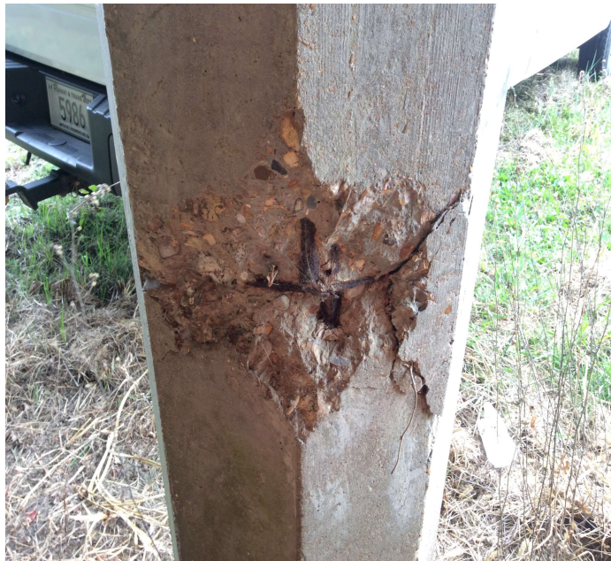
PHOTO 1 Description Spall with 1' rebar exposed to Pile 5 at Bent 2.
