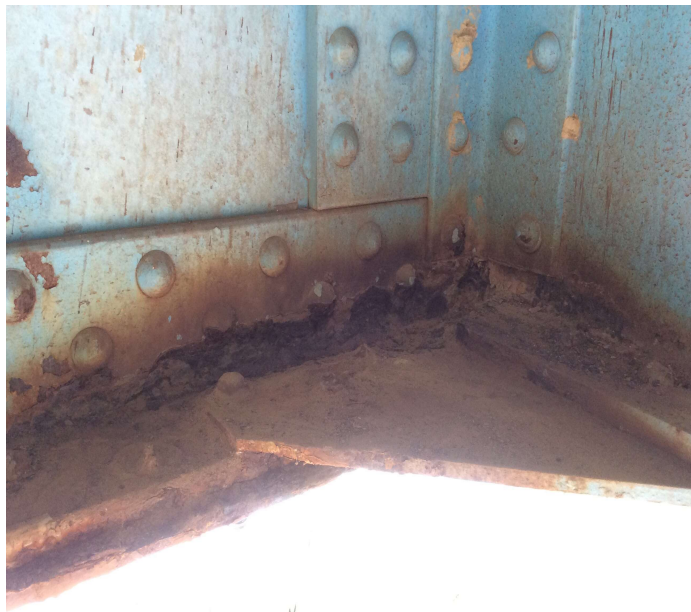
PHOTO 1 Description Heavy rust with section loss to bottom Flange of Girder 2 at Pin & Hanger 3A.
