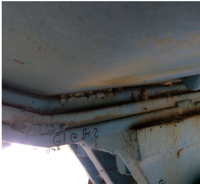
PHOTO 1 Description Cracked tack weld between bottom flange & gusset plate inside Girder #1 at end of Span #2.
