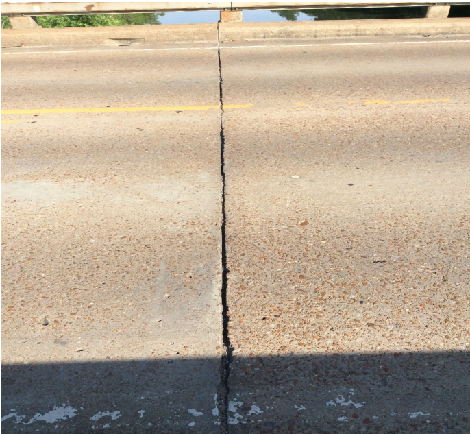
PHOTO 1 Description All Poured Joints are deteriorated & leak.
