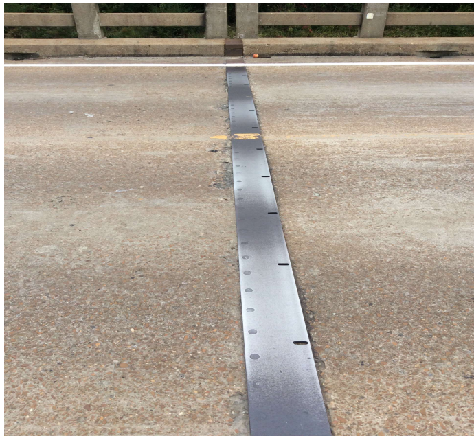
PHOTO 1 Description Spalling along sliding plate joints at Bents 1 - 4 & 6 -10.
