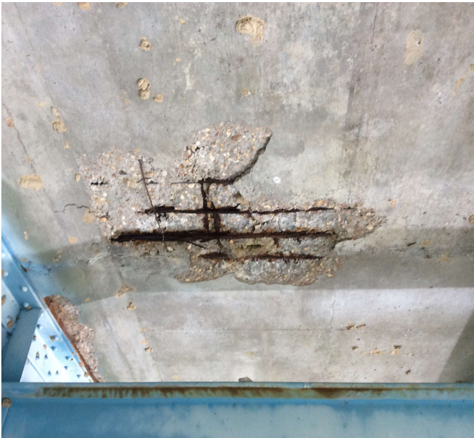
PHOTO 1 Description Span 3. Spall 12' rebar exposed to Deck below.
