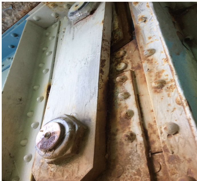
PHOTO 1 Description Pack rust @ Pin & hanger assembly 1A @ Girder 1 Span 1.
