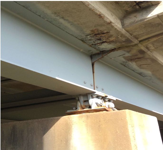
PHOTO 2 Description Typical of Out of plane bending to girders. See Form III
