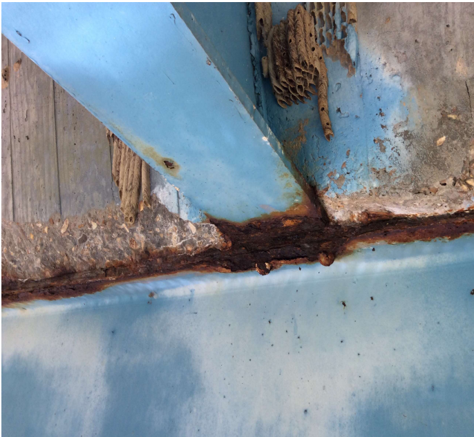
PHOTO 1 Description Span 4. Rust with section loss to top Flange of Floor Beam 3 & bottom of Stringer 1.
