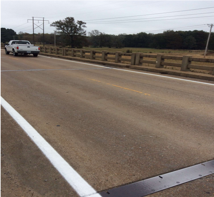
PHOTO 3 Description Typical of unsealed cracks to deck at all spans.
