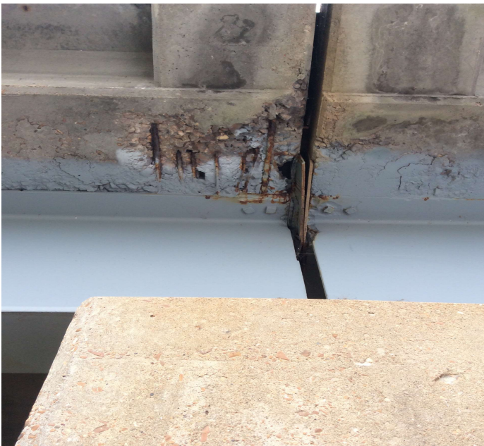
PHOTO 1 Description Typical of spalls with rebar exposed to left & right overhangs at all spans. (Bent 2)
