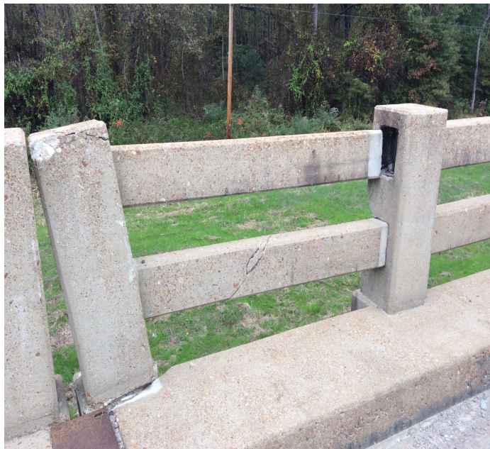
PHOTO 1 Description 1st and 2nd concrete post of left at Span 4 is broken & lower concrete rail is cracked, top rail is off post on one end.
