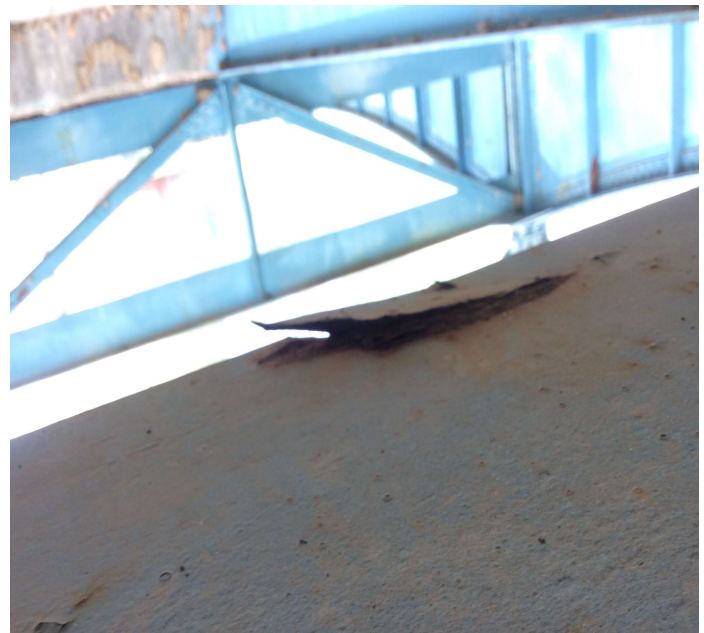
PHOTO 2 Description Floor beam 1 has a crack in top Flange at Span 5.
