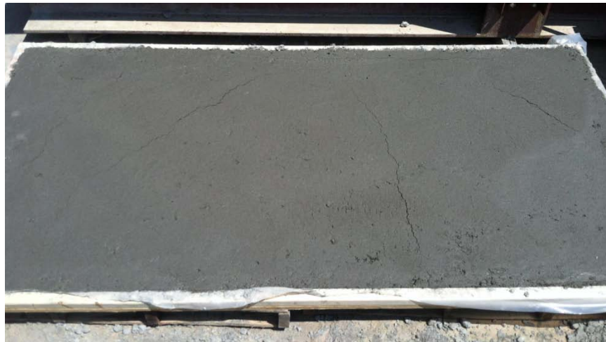
Figure 4.21 Slab After Formation of Plastic Shrinkage Cracks
