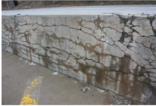
Figure 2.3-1. Example of ASR symptoms such as map cracking, cracks parallel to restraint, gel exudation, surface discoloration, etc. (Picture used with permission from Richard Deschenes).
