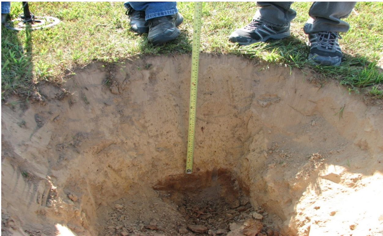
Fig. 4.2.6. A photo showing the trenching along profile no. 11 in Area 3 and the contact between the dry upper layer and the wet clay lower layer at depth of 0.51 m.
